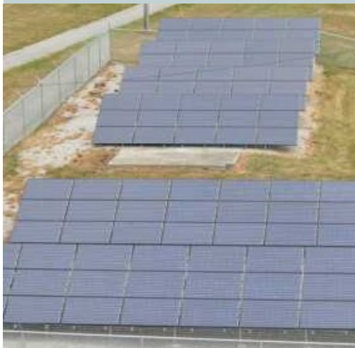
Berea Municipal Utility's Phase I and II Solar Farm
